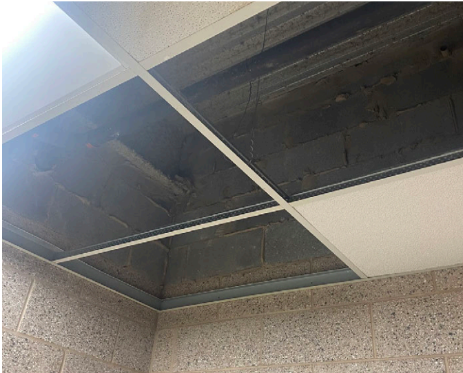
Leak in Ceiling
