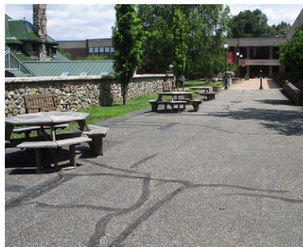
Asphalt Pavement in Poor Condition
