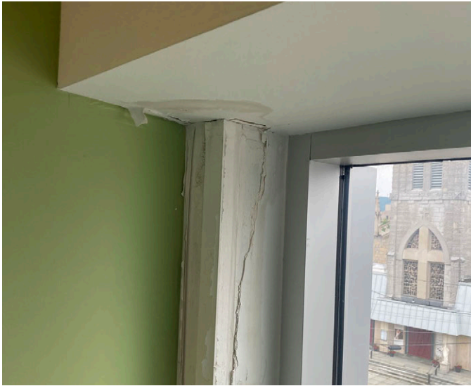
Damaged Finish in North Stairwell
