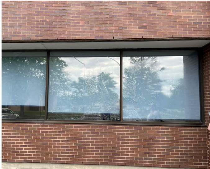
Window System in Poor Condition
