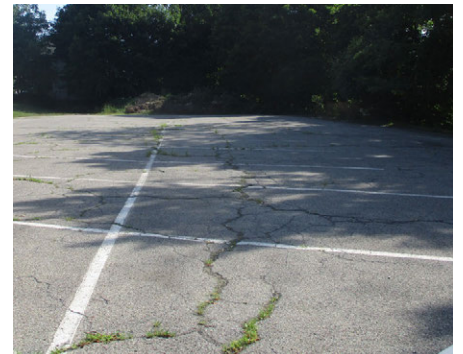
Asphalt Pavement in Poor Condition
