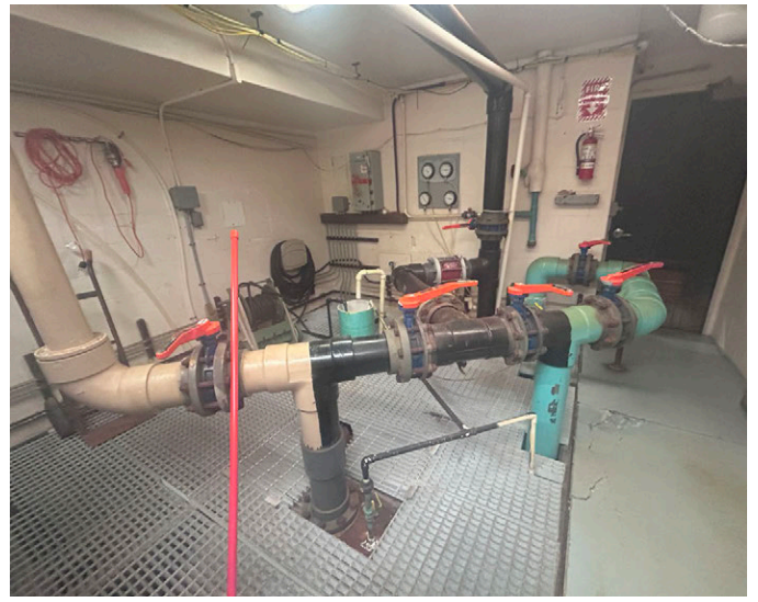
Outdated Pool Filtration System
