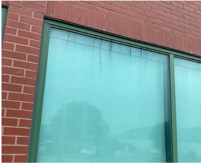
Failed Window System
