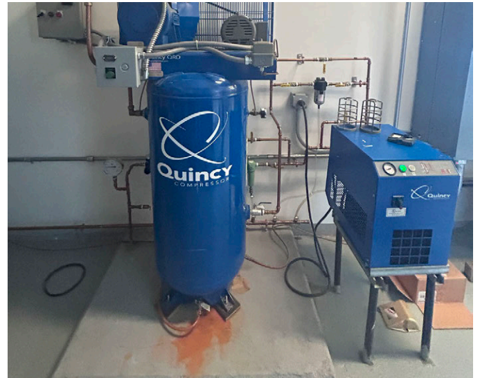
Drainage Issues at Nursing Lab Air Compressor
