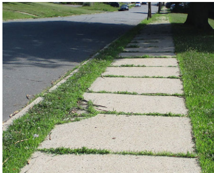
Concrete Walkway in Poor Condition
