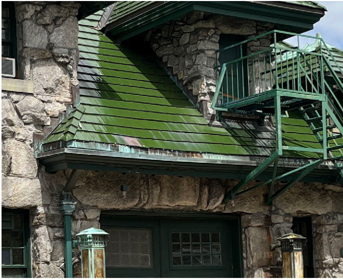
Broken Roof Tiles
