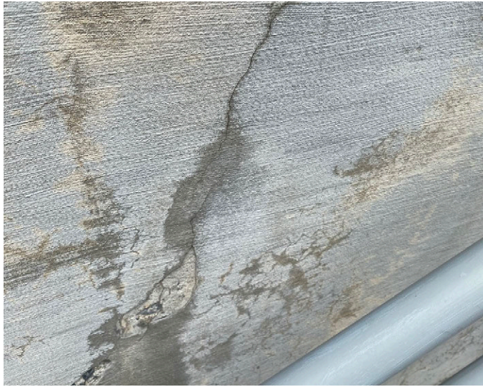
Cracked Parging at Northwest Stairwell Retaining Wall
