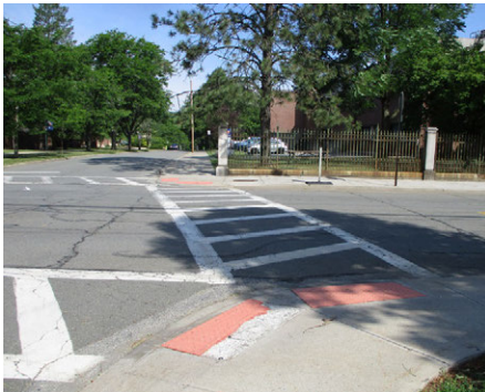
Concrete Pavement and Curb Ramps Need Replacement
