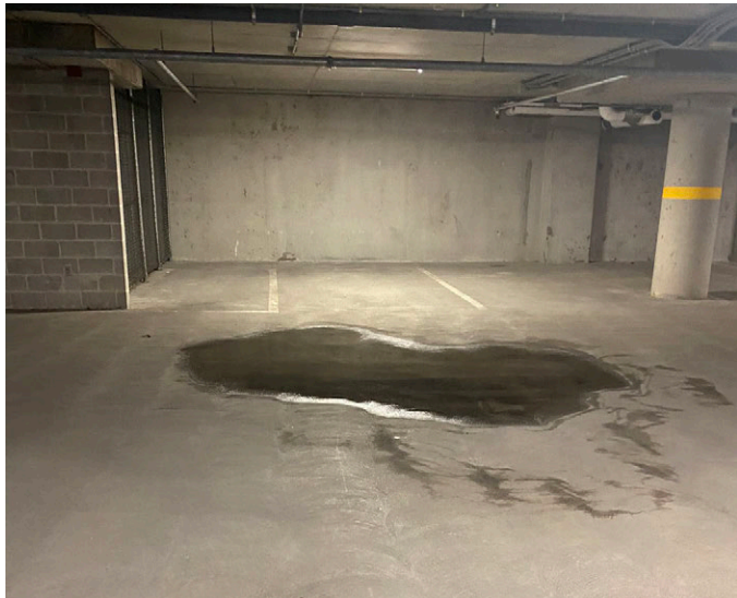
Leak in Garage
