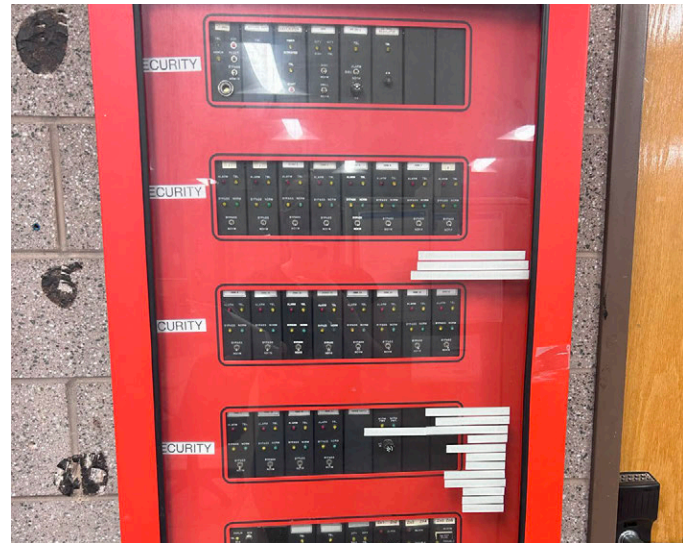
Non-Addressable Zoned Fire Alarm
