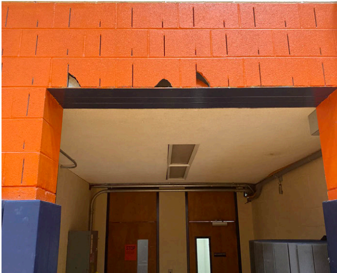
Damaged Sound-Mitigating CMU
