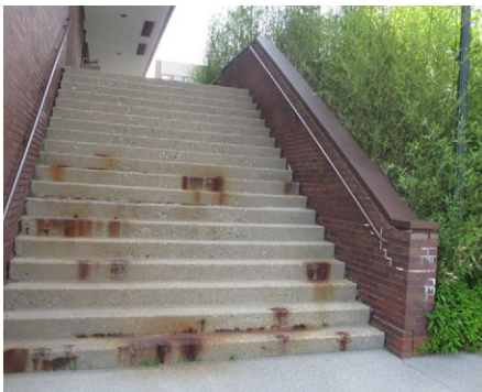
Failing Concrete Stairs Between Horton Hall and the Bio-Tech Building
