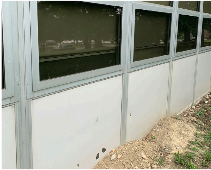
Window System in Poor Condition
