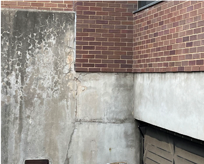
Cracked Concrete at Foundation Wall
