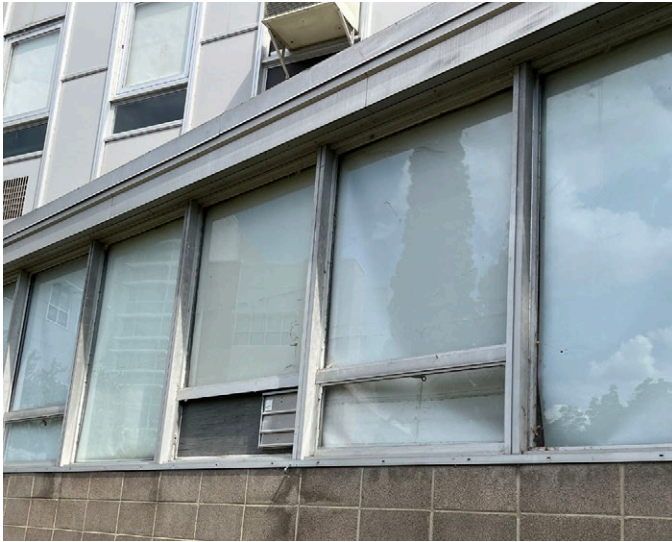
Single-Pane Windows in Poor Condition
