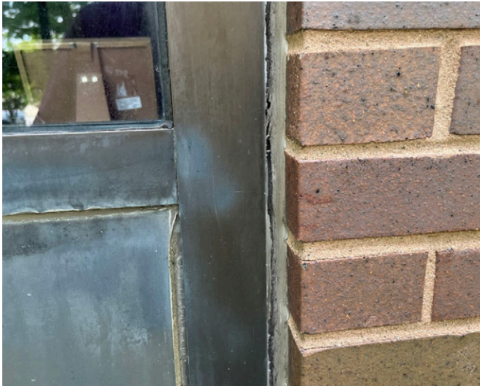
Failed Sealant at Curtainwall System
