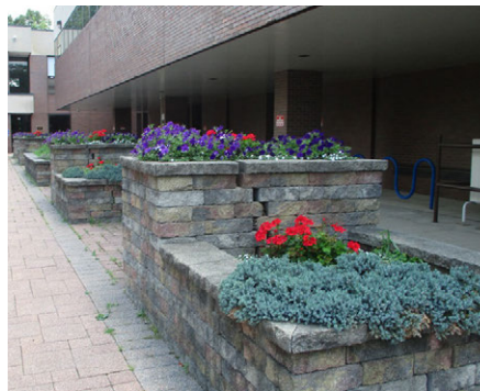
Failing Planters and Inconsistent Furnishings
