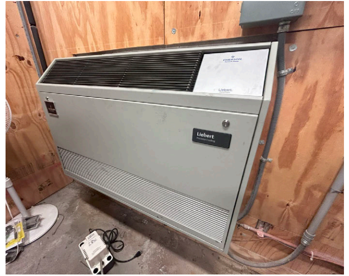
Inadequate IT Closet Air Conditioning Unit
