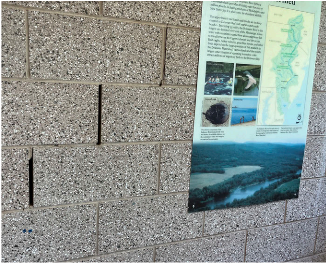
Missing Mortar at Interior Corridor Walls
