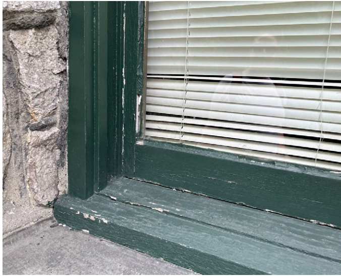
Deteriorated Window Frame
