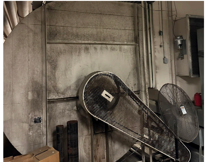
Air-Handling Unit Nearing End of Life
