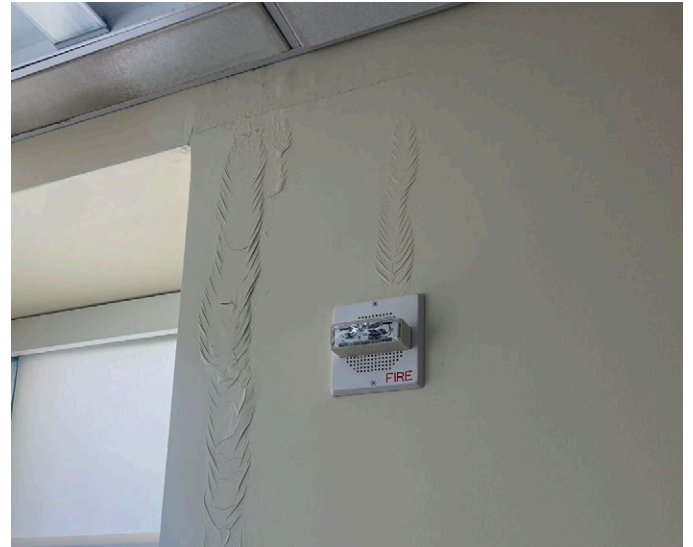
Damaged Finish in Faculty Office 415
