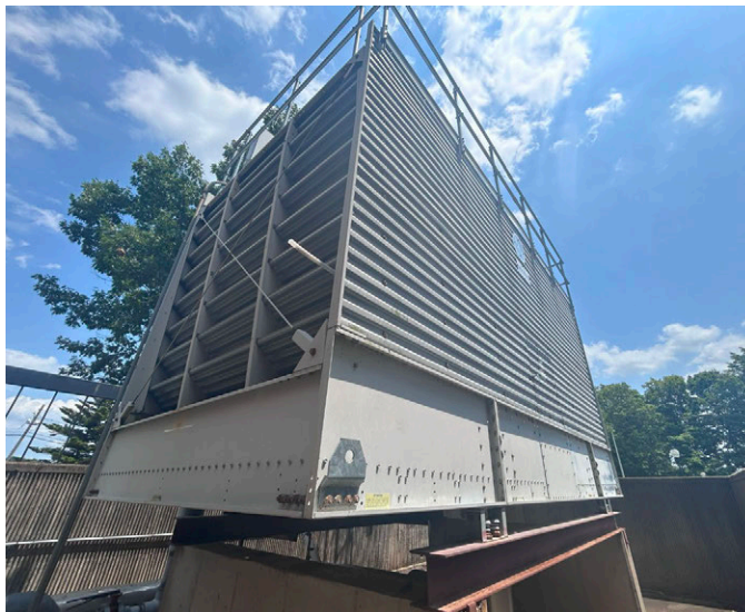
Cooling Tower Nearing End of Life
