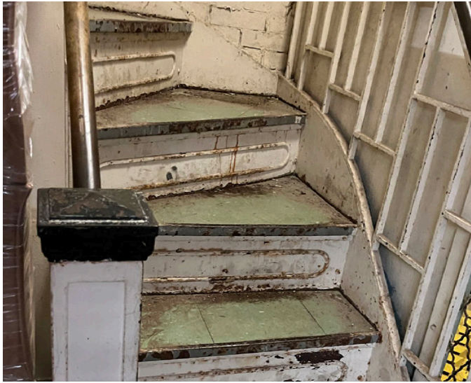
Damaged Interior Finishes
