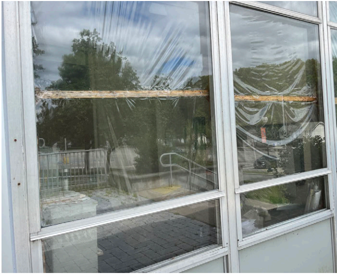
Window System in Poor Condition
