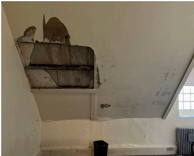
Leak at Ceiling
