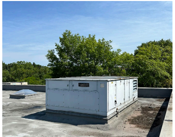
Rooftop Unit Nearing End of Life
