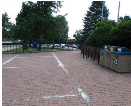
Stamped Concrete Pavement at Library Entrance Needs Replacement
