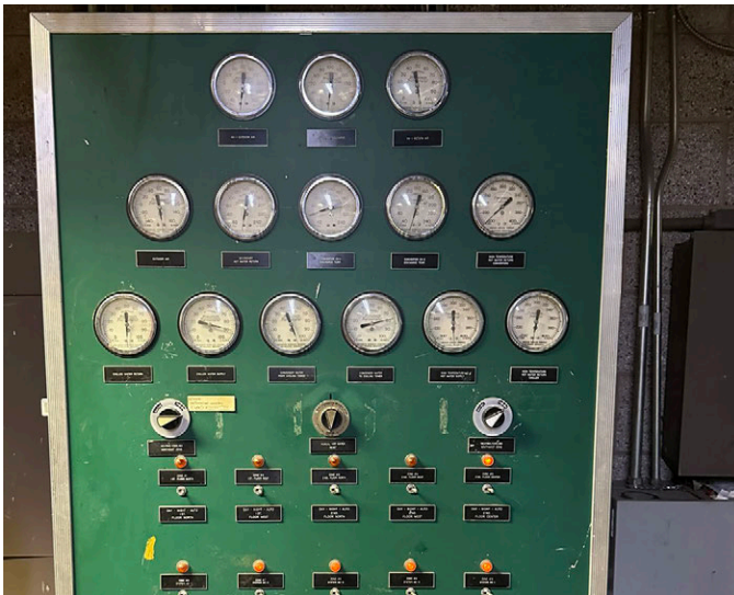
Outdated Pneumatic Controls
