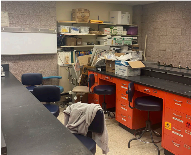
Casework in Poor Condition
