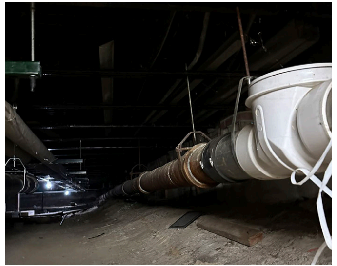
Inefficient Crawl Space Cleanout
