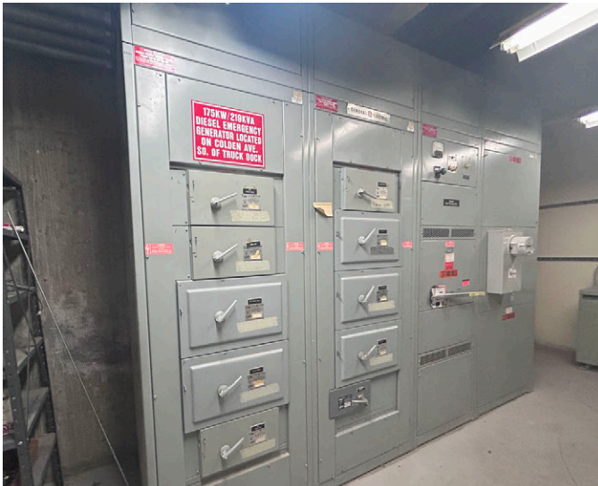
Original Electrical Distribution Equipment Needs to be Replaced
