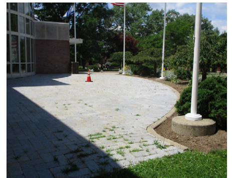
Differential Paver Settlement at Plaza North of the Library
