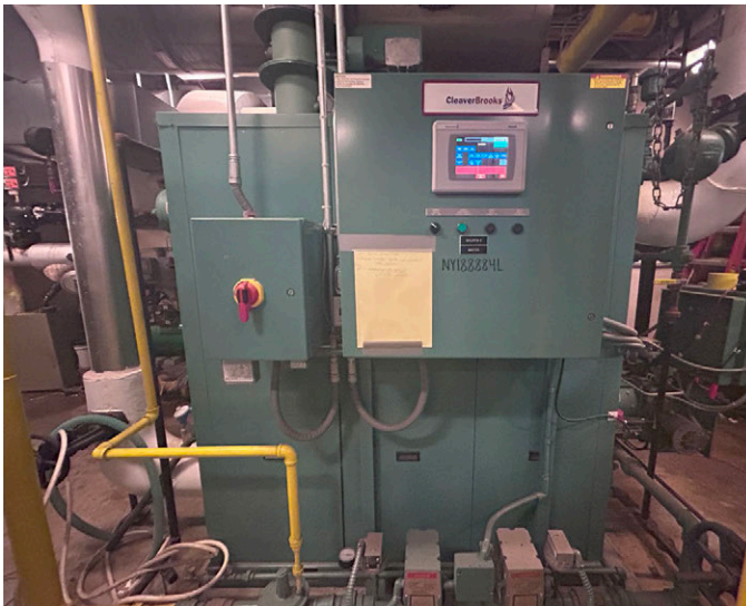
Boiler Nearing End of Life
