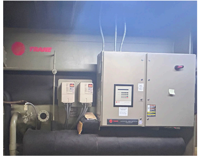
Chiller Nearing End of Life
