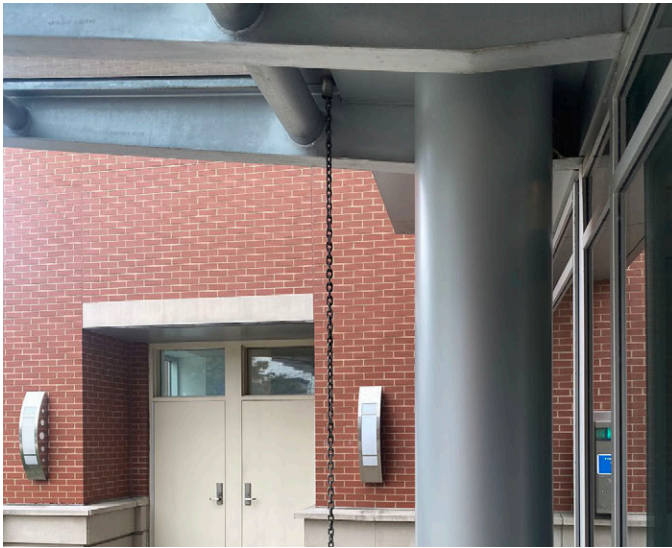
Infiltrating Water at Rain Chain at Entrance
