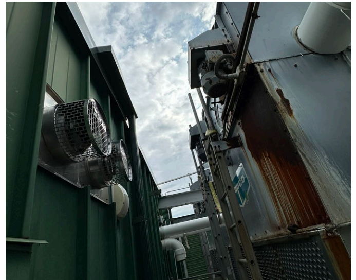
Rusting Cooling Tower
