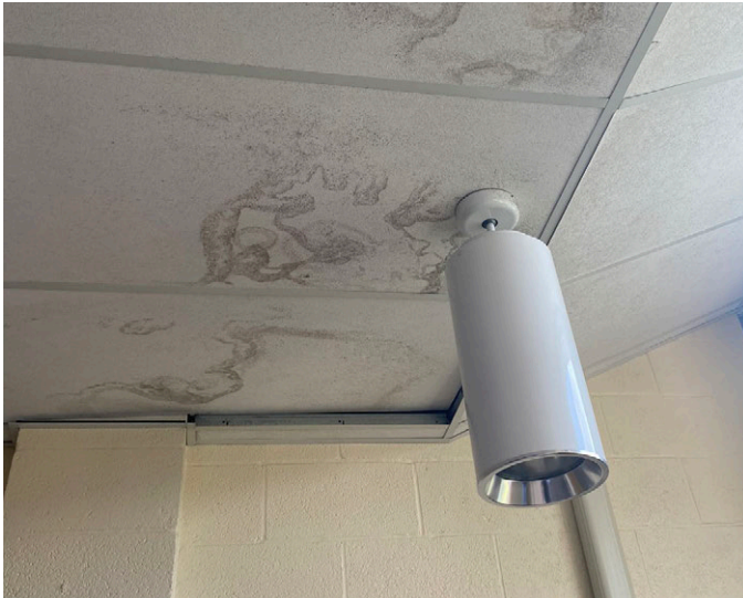
Damaged Ceiling Tiles
