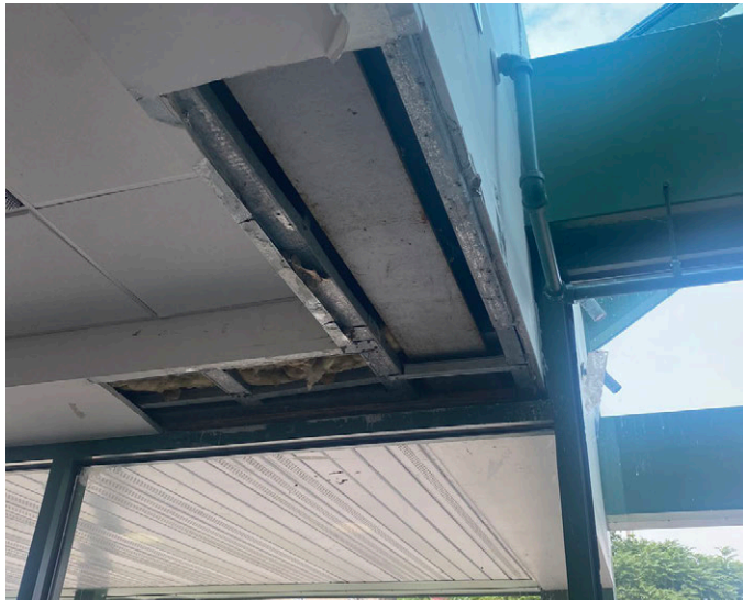
Damaged Ceiling in Lobby 100
