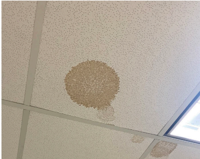
Damaged Ceiling Tiles
