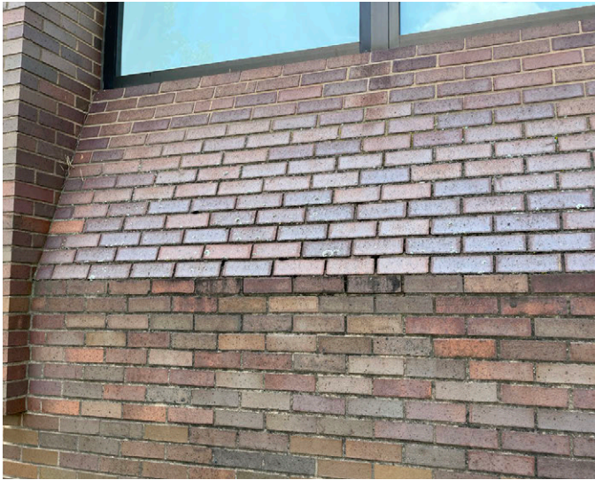
Deteriorated Masonry at Windows
