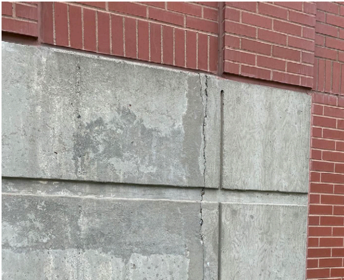
Cracked Foundation Wall
