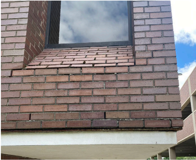
Deteriorated Mortar Joints
