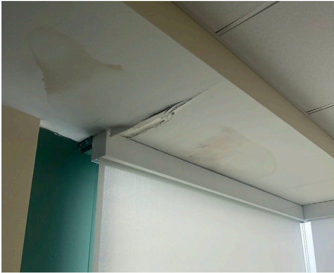
Damaged Ceiling in Faculty Office 415
