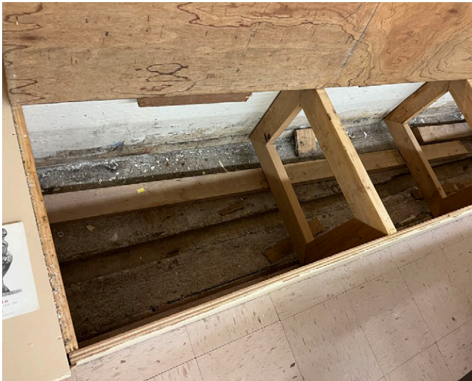
Inefficient Gutter at Student Lounge
