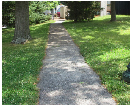
Walkway Not Accessible due to Excessive Slope
