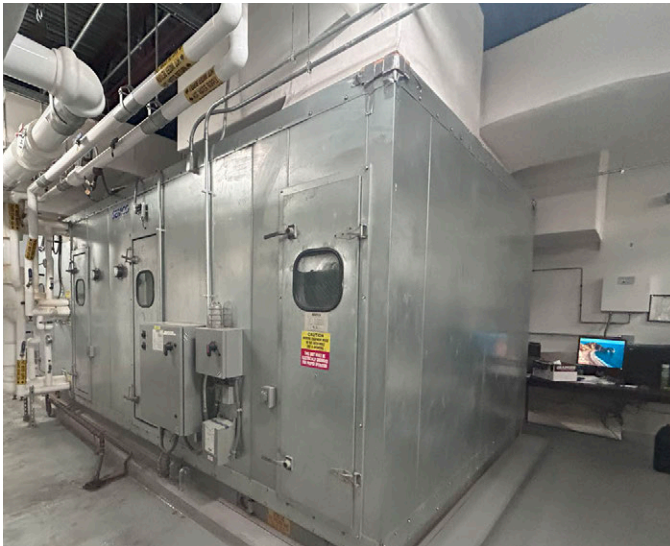
Failed Air Handling Unit Motors
