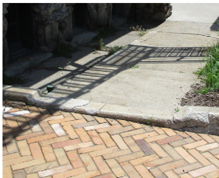
Differential Settling of Pavement Materials
