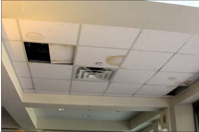
Damaged ceiling tiles should be replaced.
