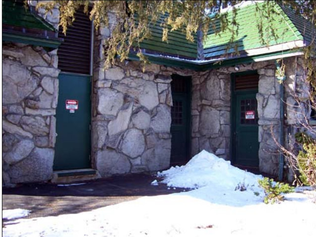
Snow falls from the roof and piles up in front of the building's two secondary doors. The main door to the upper floor is seen on the left.
