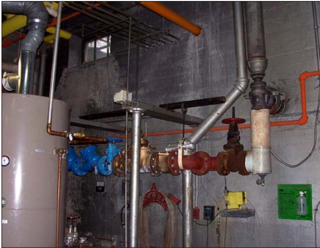
Water service entrance.
