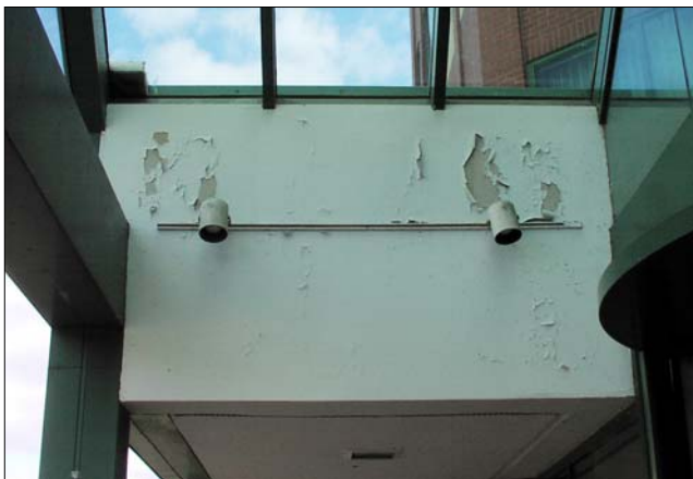
Exterior soffits need to be repainted.
