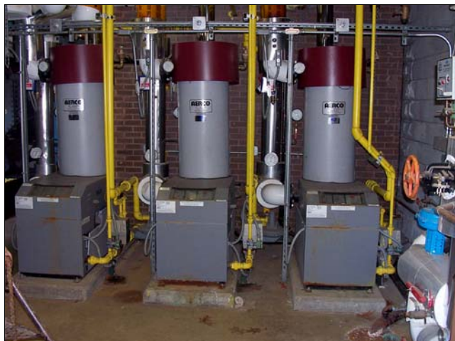
The boilers were recently replaced.
