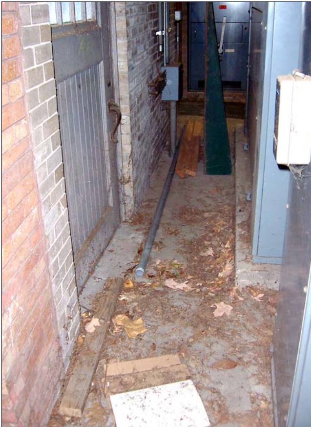
Dirt, leaves and other debris found throughout the upper floor of the building can infiltrate the transformers as there are no filters on these older units.
