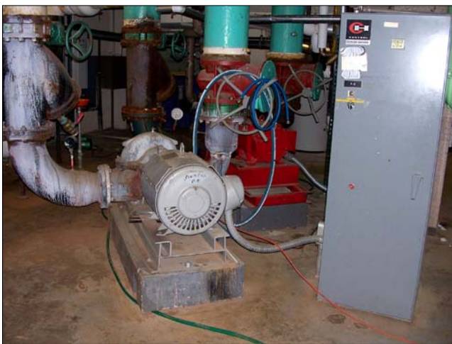
The existing tower pumps should be replaced.
