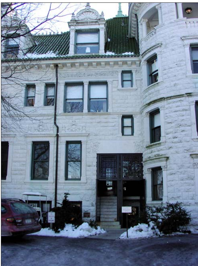
Snow and ice falling from the roof pose a potential hazard to pedestrians below.
