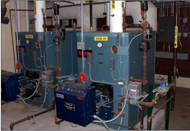
New boilers were recently installed.
