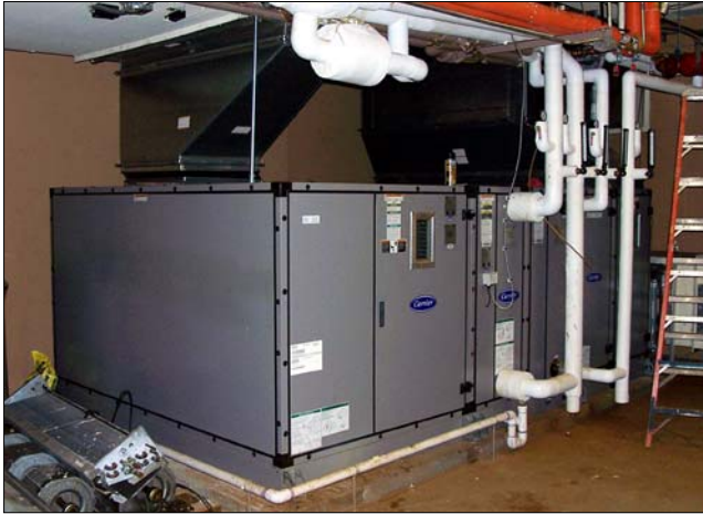
New air-handling unit located in the basement.
