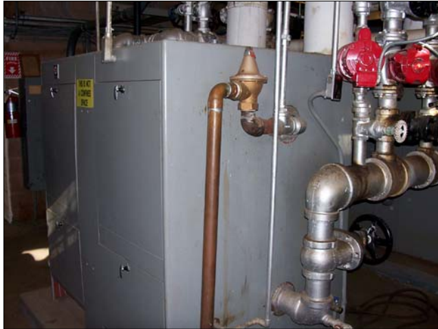
The two old boilers should be replaced.
