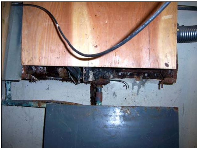
The rusted cover of an electrical panel has been replaced with a piece of wood. The building's entire electrical distribution system should be replaced.
