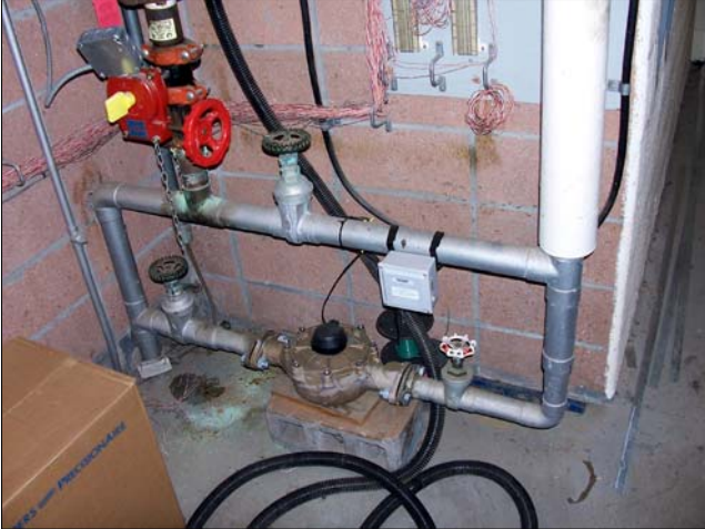
A backflow preventer should be installed at the boiler connection to protect the domestic cold water system.
