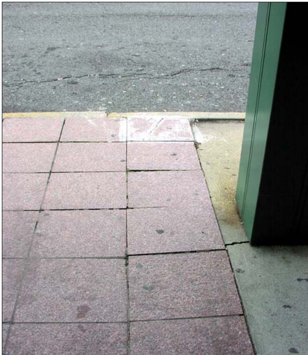
Damaged and heaving sidewalks and curbing should be repaired or replaced, as needed.
