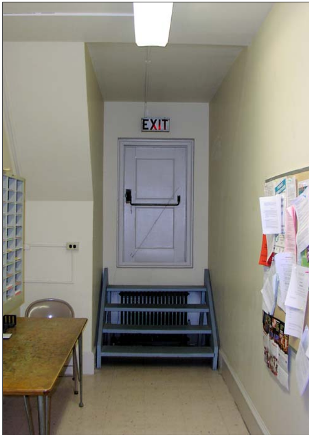
The second means of egress from the upper floor is via a 57" high door that leads to a fire escape. The College should construct an additional, code-compliant means of egress to serve the upper floor when the building is renovated.
